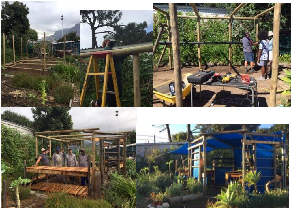
First the ground to be levelled, then poles to be sunk, Then uprights.. Thank goodness we had Gary & Lizzy who managed to keep the guys on track!
